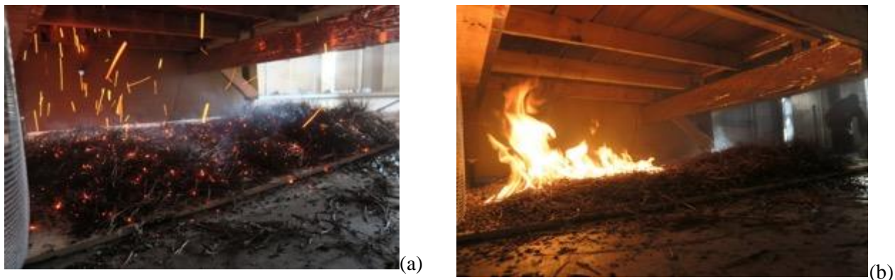
Figure 3. Ember penetration through gaps between deck boards; (a) embers falling to ground and (b) resulting in the ignition of pine needles that accumulated under the deck.
